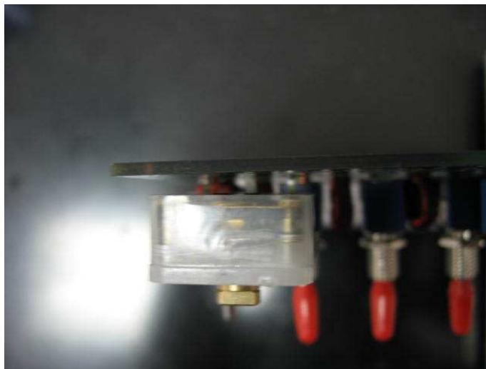
Figure 10 – Note gap between board and polyvaricon
